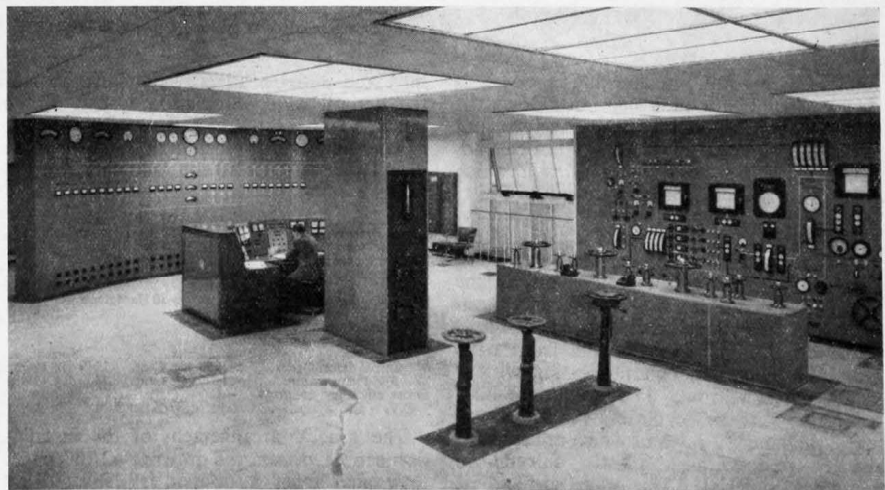
Steam and electrical control room at Kynoch works power-house
